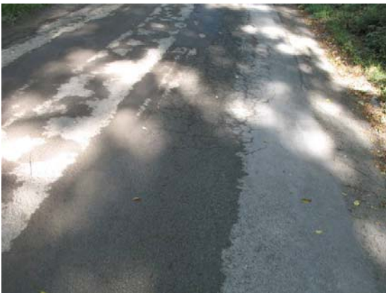
Alligator cracking and patch
