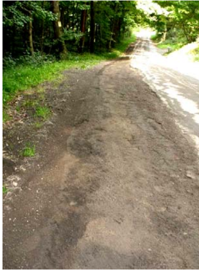
Downhill view, deteriorated shoulder
